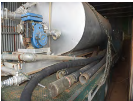
Lot: Water Tank & Pump
